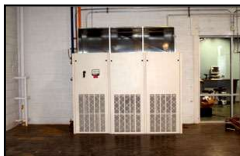
An A/C Unit Cooling the Server Area
