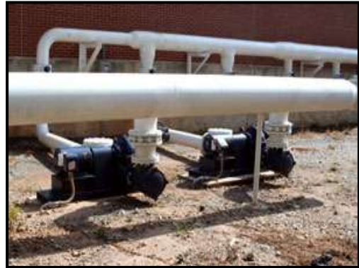
Water Pumps Fueling the A/C Units
