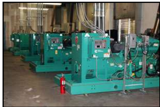
Backup Power Generators
